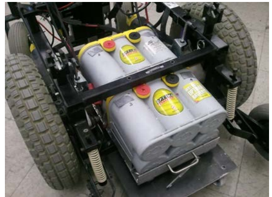
Figure 3.1 Fabricated Battery Tray
